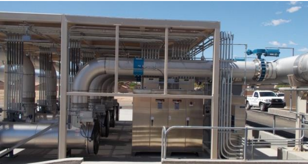
Advanced Treatment Systems
