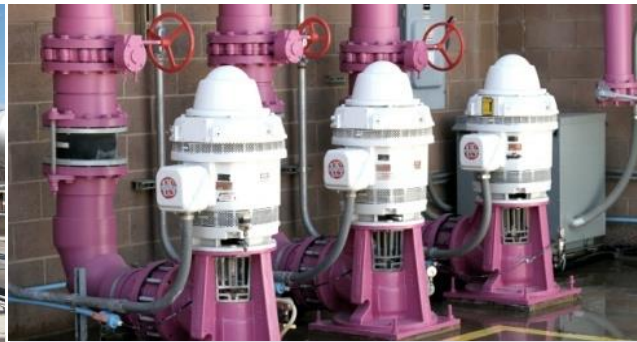
Automated Asset Management
