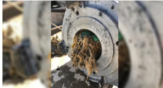
That's wet wipes clogging up expensive equipment at the Global Water Resources, not to mention creating a mess for treatment plant employees.
